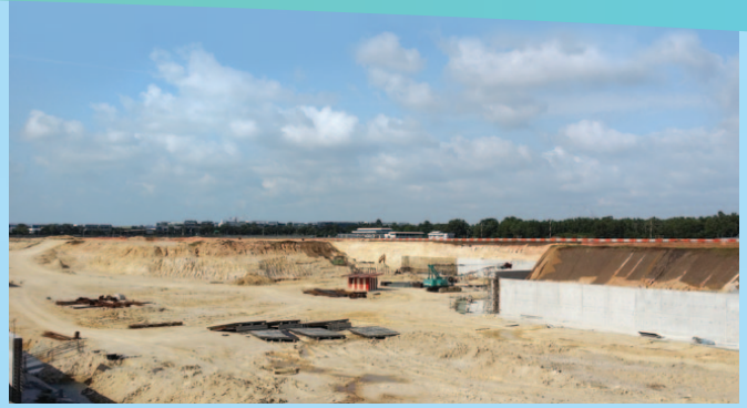
THE NEW RESERVOIR BEING CONSTRUCTED. ITS WATER HOLDING CAPACITY WILL BE THREE TIMES LARGER AND FITTED WITH PUMPS FOR BETTER FLOOD PREVENTION
